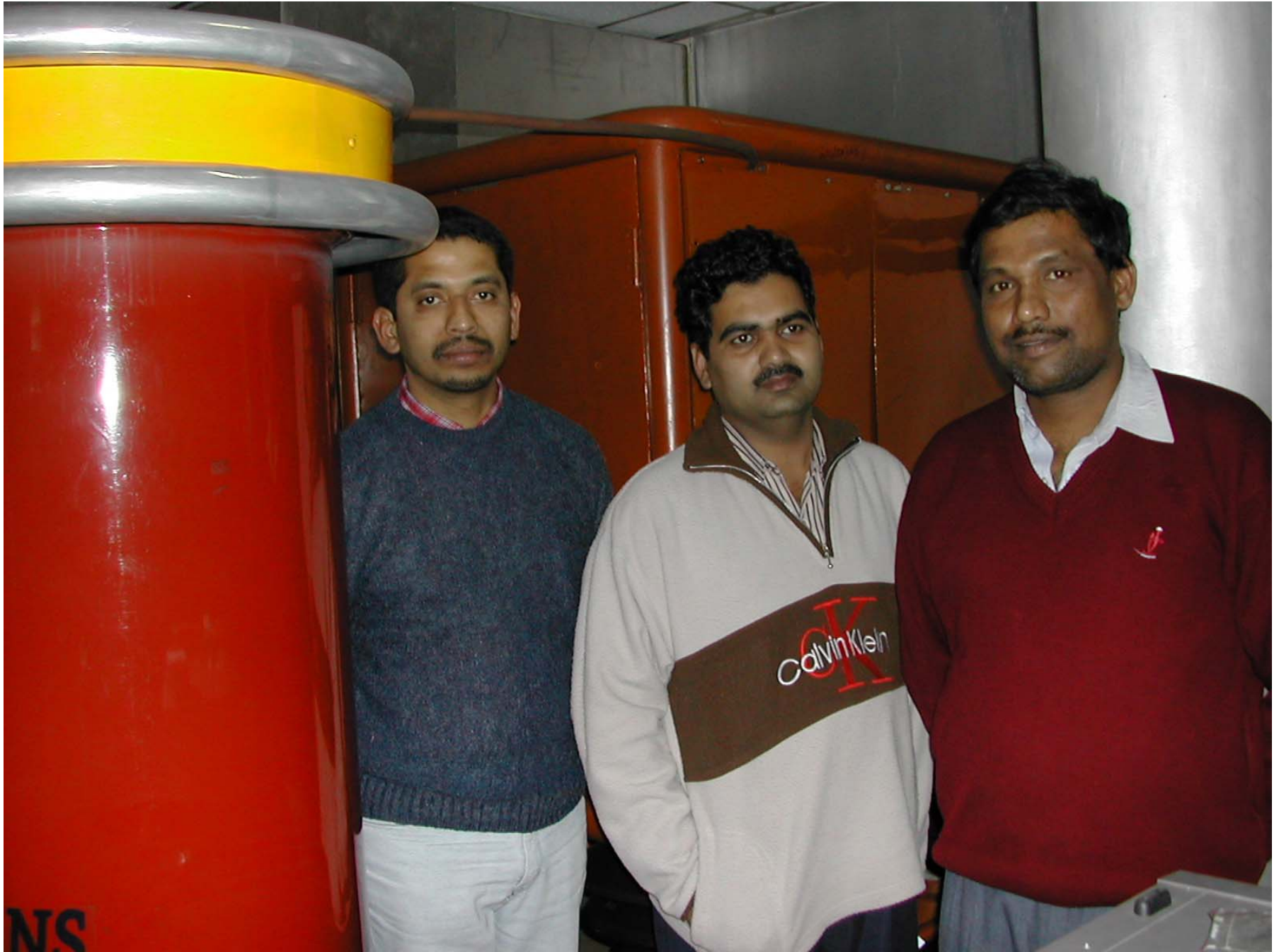
Isolation Transformer supplying power to the HV platform
